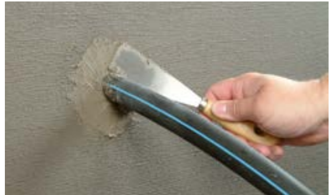
In order to protect the waterproofing and provide mechanical support, the area around the pipe or cable is plugged with KÖSTER KB-Fix 5.
