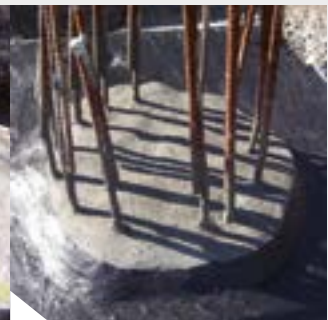
Connection of the area waterproofing (KÖSTER Deuxan 2C) to the pile head waterproofing.
